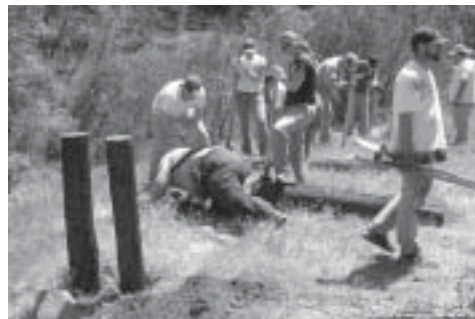
Volunteers rebuilt miles of fences, restored trails, replaced signs and made a large portion of the park safe enough to reopen.
